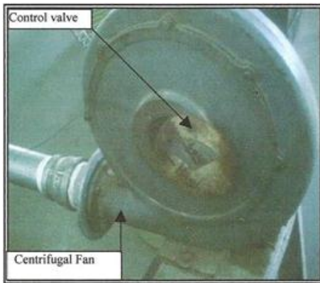
Figure 8: Centrifugal Blower and Control Valve.
