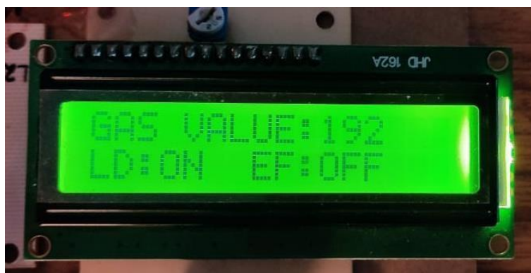
Figure 5: The gas level displayed on LCD before gas leakage
