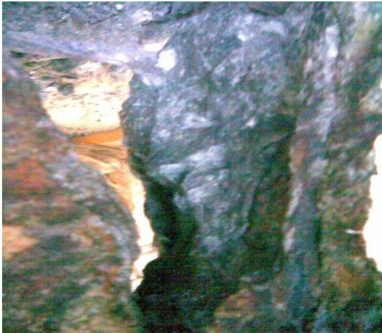
Fig. 6 The failure pattern and the effect of corrosion
