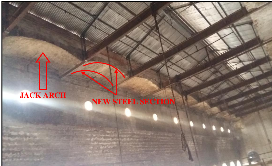
PLATE 1 : VIEW OF JACK ARCH MADE WITH BRICK MASONRY AT TURNING SHED. STEEL SECTION IS TO BE WELDED AS PER SKETCH.
