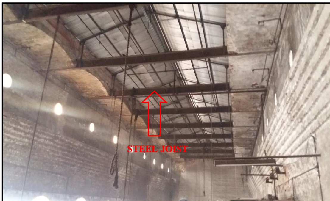
PLATE 2 : VIEW OF CORRODED STEEL JOIST.
