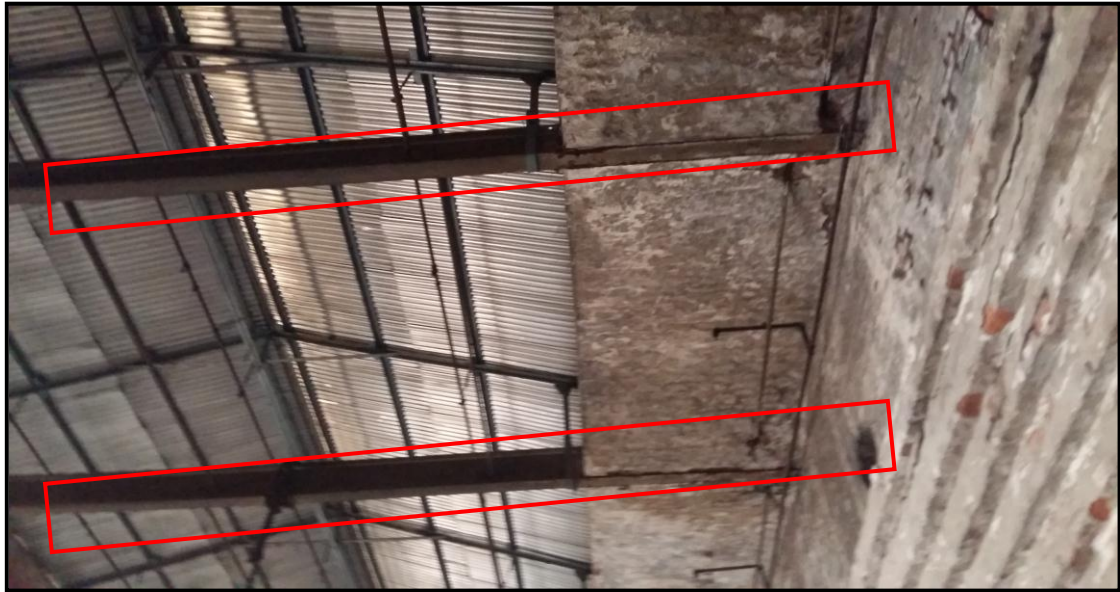
PLATE 3 : MODERATE CORROSION AT STEEL JOIST.
