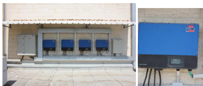
Fig. 3. Photo of the considered inverter.
