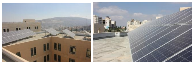
Fig. 2. Photo of the installed PV array at roof top of Engineering Faculty building.
